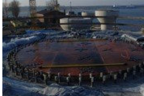
Fig. 10: Position of mounting bolts in the concrete foundation and preparations for the measurement
