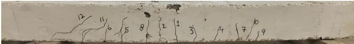
Fig. 5b. Crack Propagation of RC beam using Hybrid Reinforcement(H30 0PVA)
